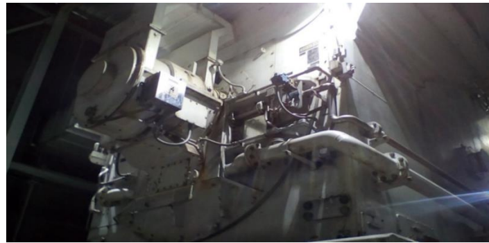
Figure 1. Gas Generator-Alternator assembly.
