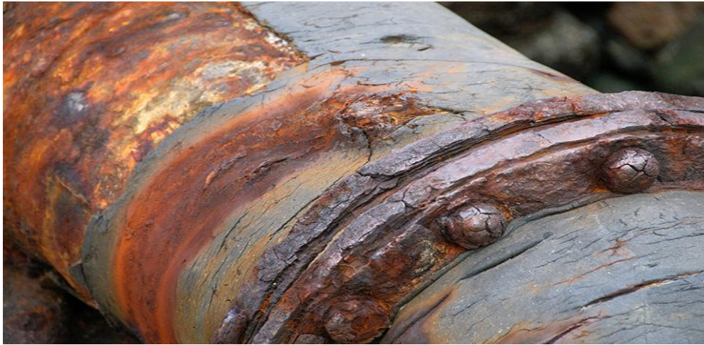
Figure 4: Stress Corrosion Cracking in Oil and Gas Pipelines in a Corrosive Environment
